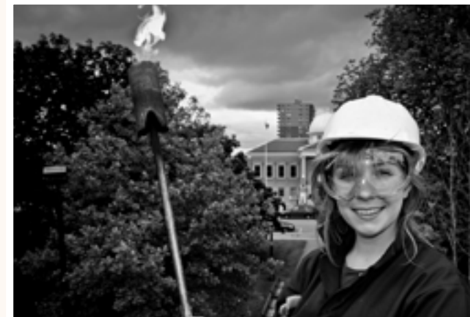
Photo: Brittany standing in a boom lift, ready to heat the bronze statue. Photo by A. Gabov, 2013.
