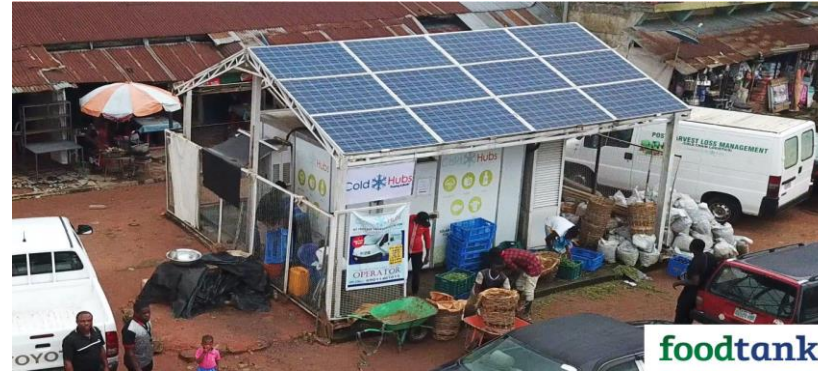
Solar-Powered Cold Storage Facility, NIGERIA
